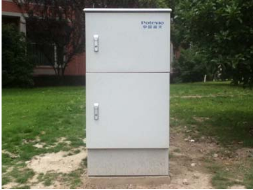
Figure 2 Charging pile integrated cabinet Electric vehicle data communications network platform frame shown in Figure 1. Pure electric cars and charging network access points will pile charging piles arranged in the vicinity, which is placed in the charging piles integrated cabinet (Figure 2) in. Integrated charging piles around the cabinet will be available through the vehicle charging piles internal wireless routers get connected to the wireless network, the router will also share their Internet connection to the vehicle users, and charge pile. Here, the router to get Internet connection, there are three main ways, one through a wired network (fiber-optic network, ordinary broadband networks, dedicated networks, etc.) to obtain Internet network connection, the second is to get Internet via 3G cellular networks network connection, three by 4G cellular network of Internet network connection. Pure electric car charging pile and can be obtained through these networks link the ability to connect with a remote server, allowing the recorded data itself is sent to the remote server database. Based on these data the remote server, you can think that pure electric car manufacturers to provide various customized data services.
